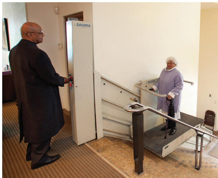
A chair lift will assure people with disabilities that their presence and their gifts are welcomed in the parish.
